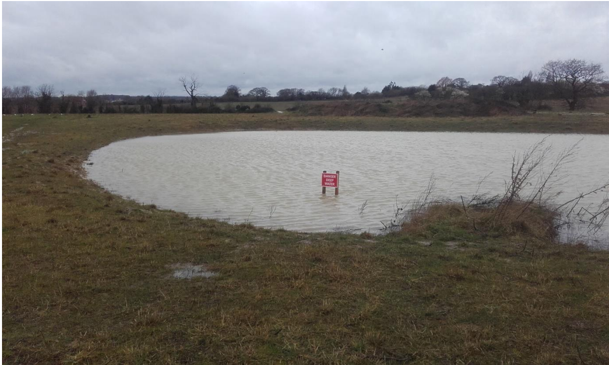
Sustainable Urban Drainage System ( S.U.D.S. ) Feb 2020
